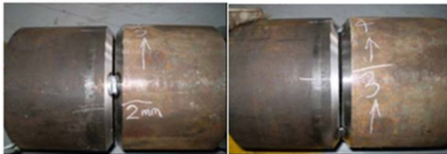
Gap between 2~6mm and miss-alignment between 0~2mm
